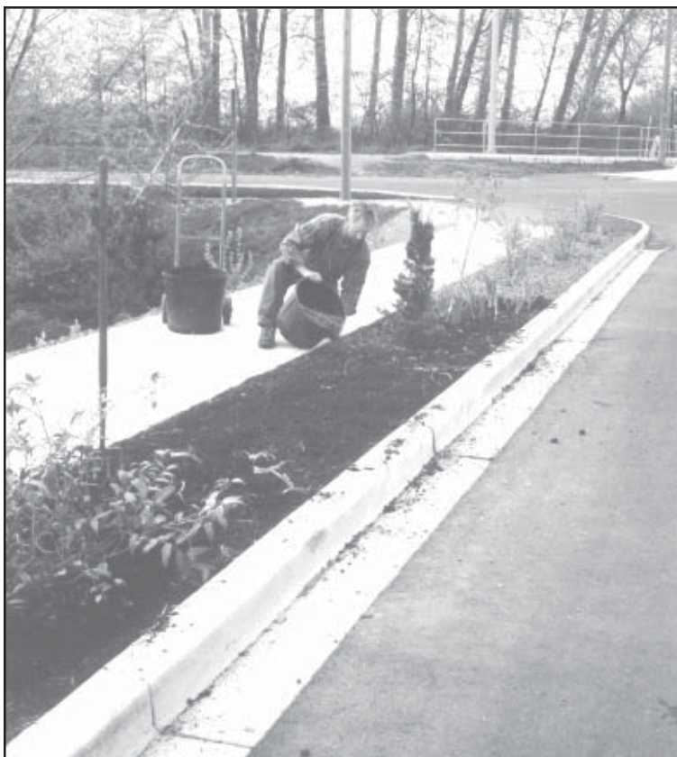
Application of wood chips onto boulevard strip between sidewalk and road. Plantings there include vine maple, saskatoon, Indian-plum and highbush cranberry.
